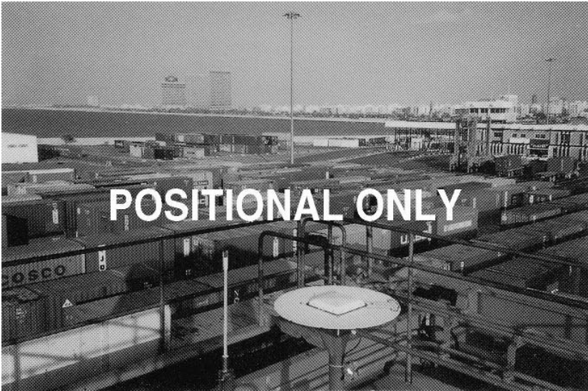
Fig. 6.9.1 DGPS antenna on a straddle carrier
