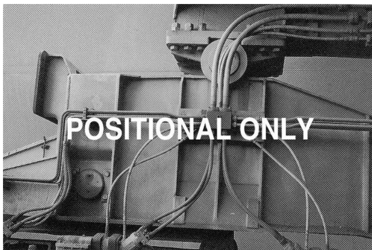
Fig. 8.4.5 Feeding the crane travelling motors of Fig. 8.4.4
