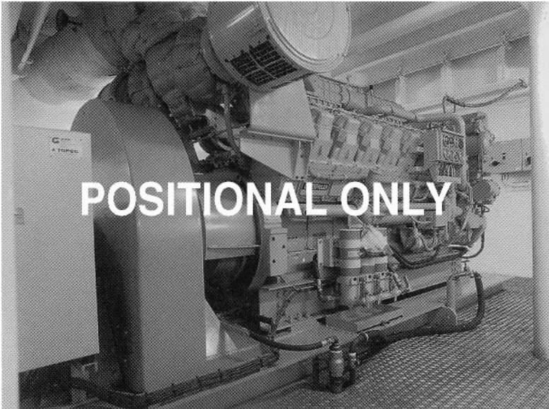
Fig. 3.9.4 Caterpillar diesel generator set with large flywheel
